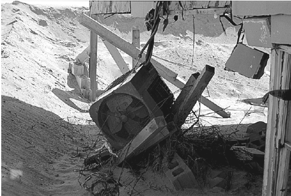
Figure 3.1.3A: Electric heat pumps dislodged from their stands by velocity flow during Hurricane Fran in Topsail Beach, North Carolina, in November 1996
