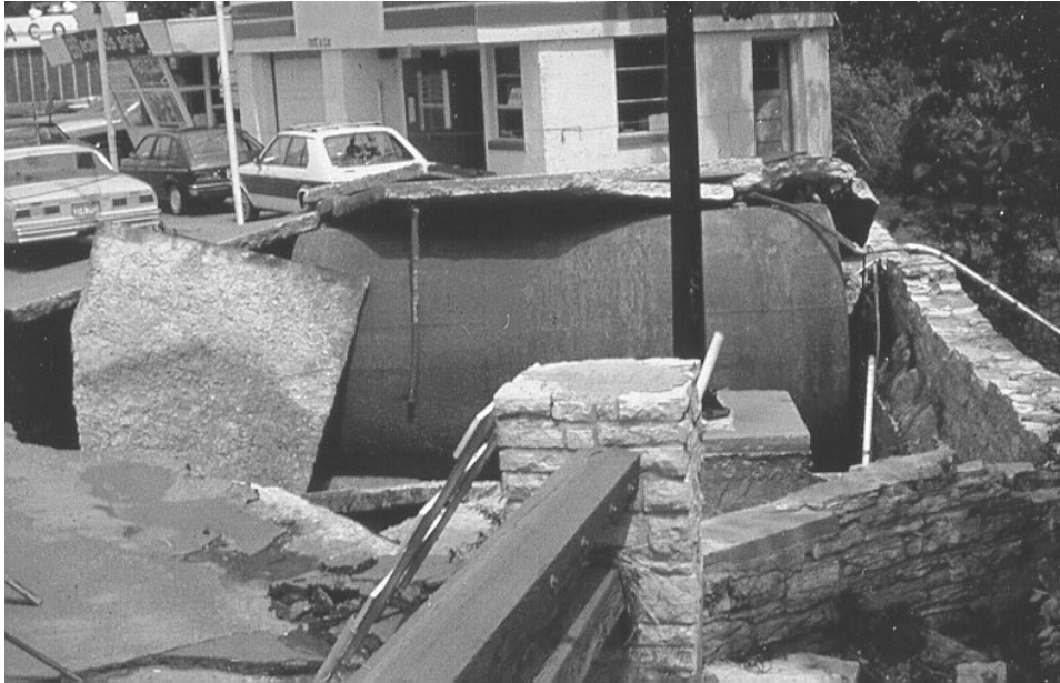
Figure 3.2.3.1A: Tank lifted by buoyancy forces
