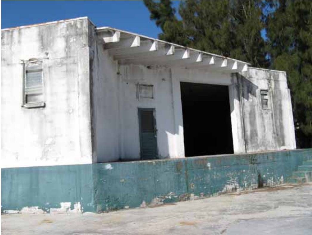
Building kept for restroom, park equipment storage and working green building demonstration site
